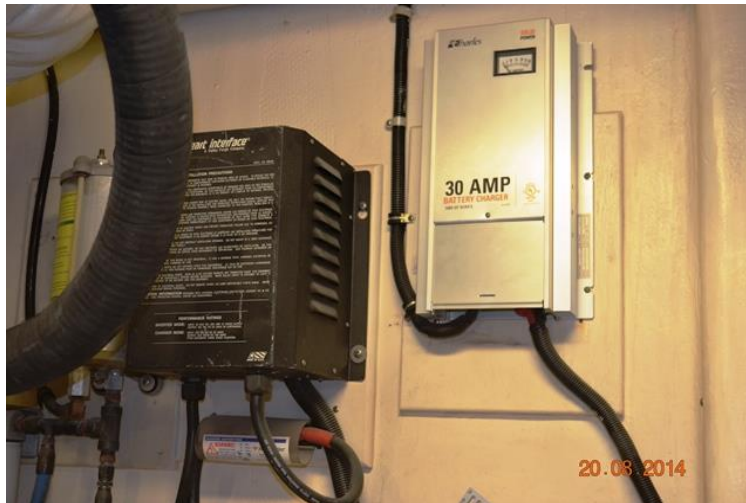
INVERTER & A BATTERY CHARGER
