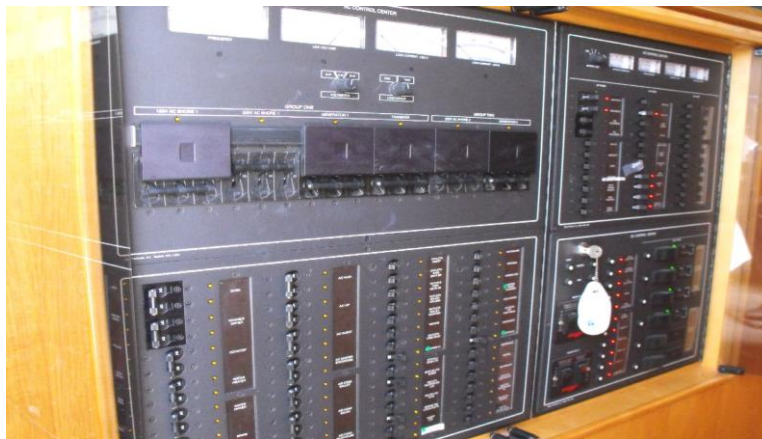
MAIN ELECTRIC PANEL
