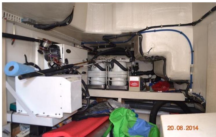
AIR CONDITIONING UNITS
